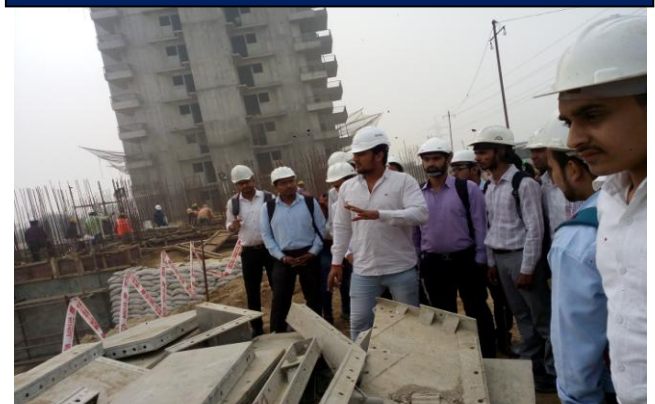
Site Engineer explaining about the Mivan shuttering and Foundation Layout Work to the Students
